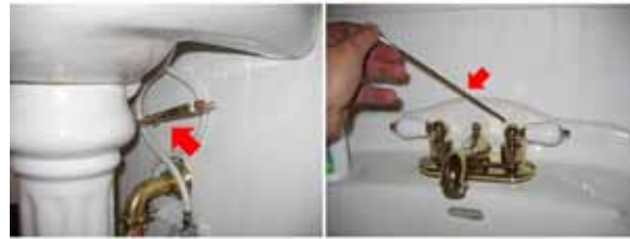
Inoperative vanity sink stopper
