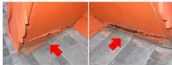
Loose roof flashing - Gabel corners
