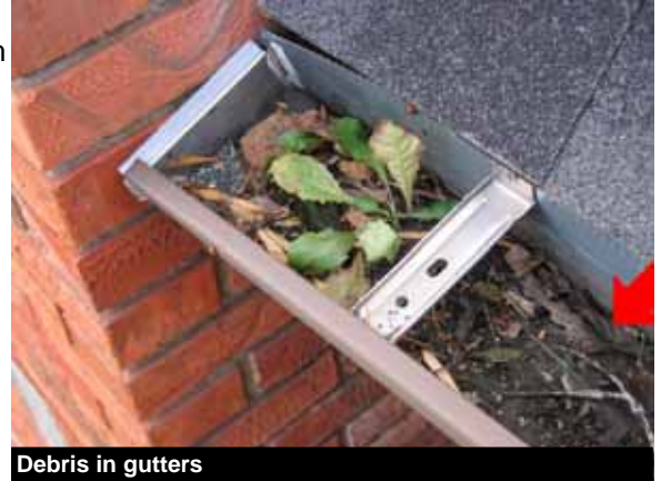
Debris in gutters
