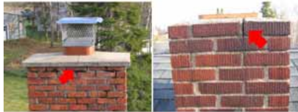
Cracked Caps and Flacking brick
