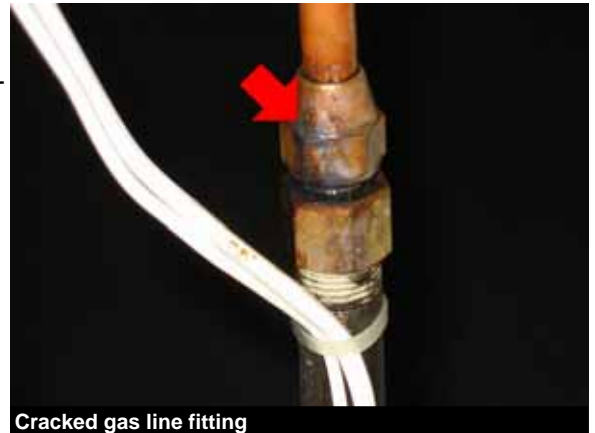
Cracked gas line fitting
