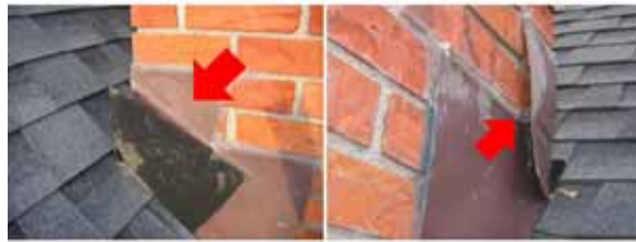
Loose chimney flashing
