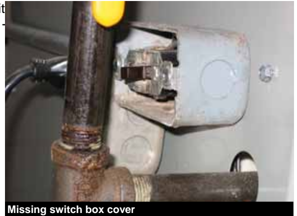
Missing switch box cover
